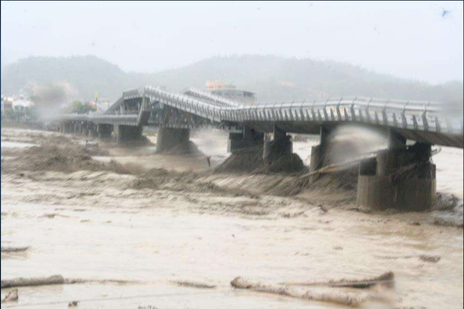
This bridge was destroyed by Typhoon Morakot in Qishan, Kaohsiung. Photo by Tang Chiang-Hu August 9, 2009
