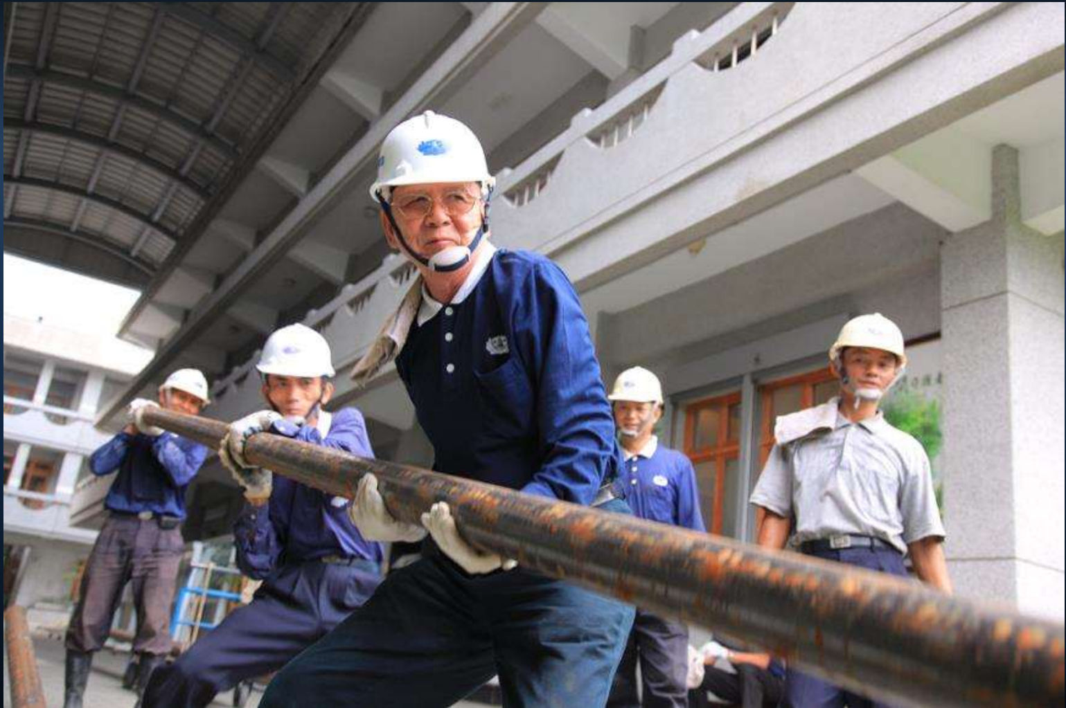
The construction of Jing Si Abode in Hualien. Photo by Hsiao Chia-Ming October 20, 2009
